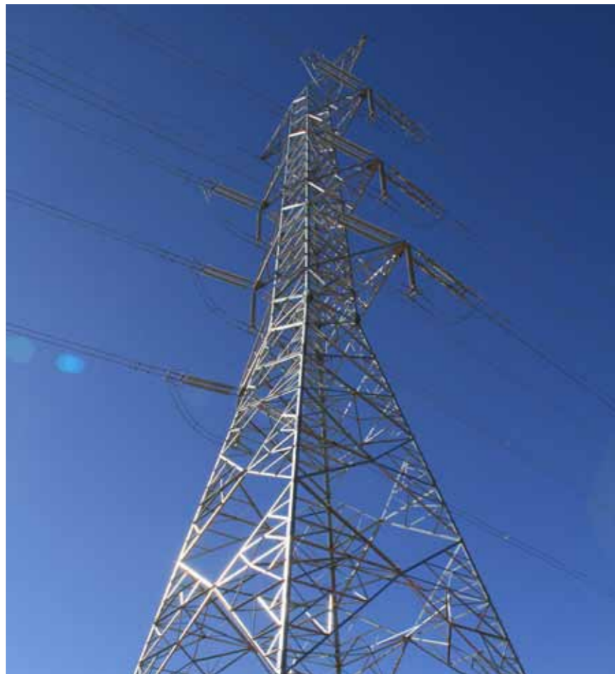
330kV transmission line, Three Springs
