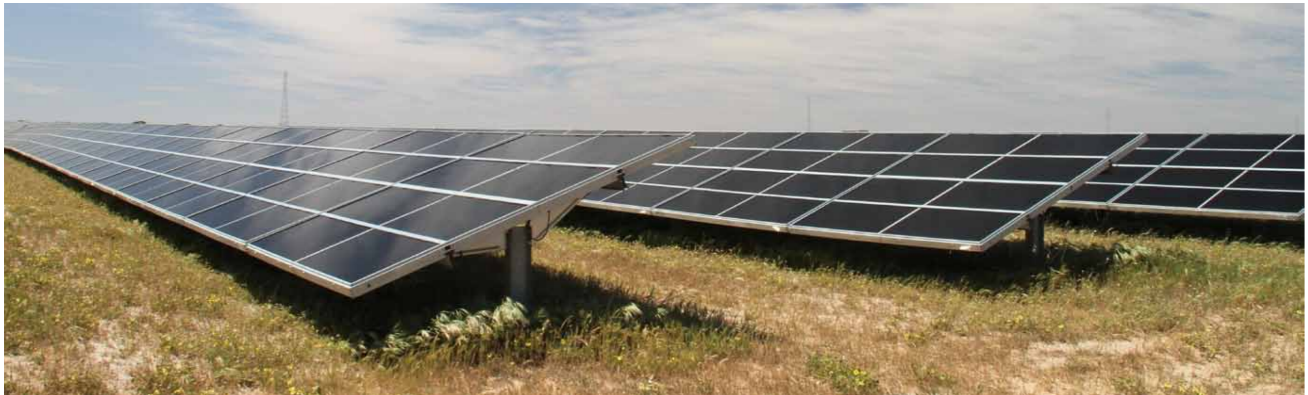
Greenough River Solar Farm, Walkaway
